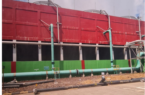
Area Power Plant (power block) PLTP Patuha Unit 1.
